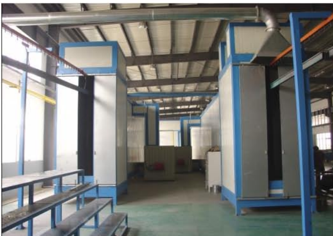
Dry off oven & curing oven
